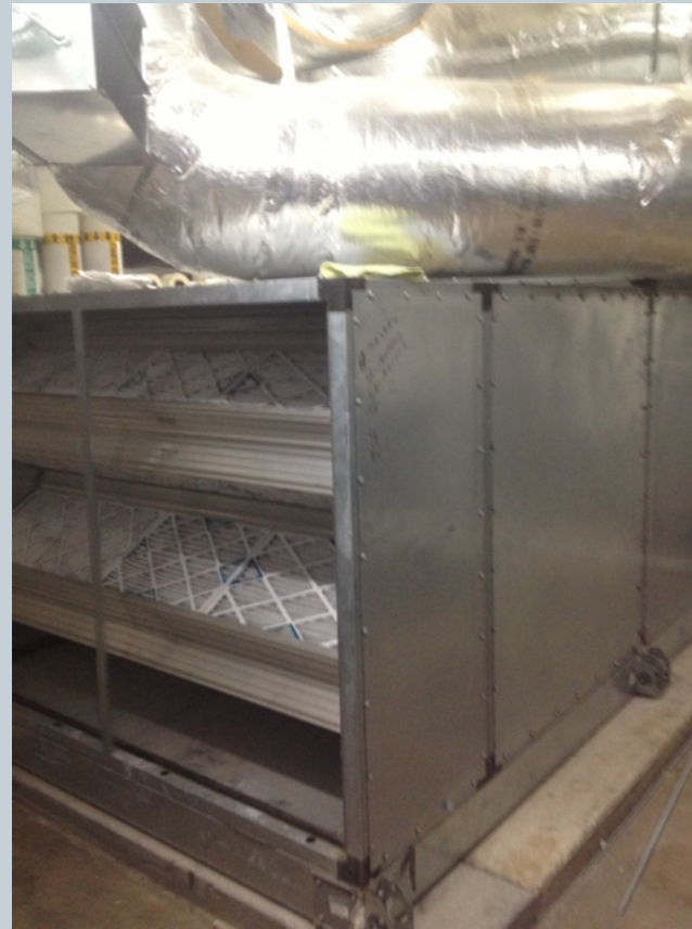
AIR HANDLING UNITS
